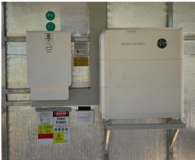
Pictured: The new battery system at Humpty Doo Community Garden.
