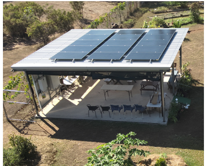
Pictured: The Humpty Doo Community Garden solar system and battery installed on the shade structure.
